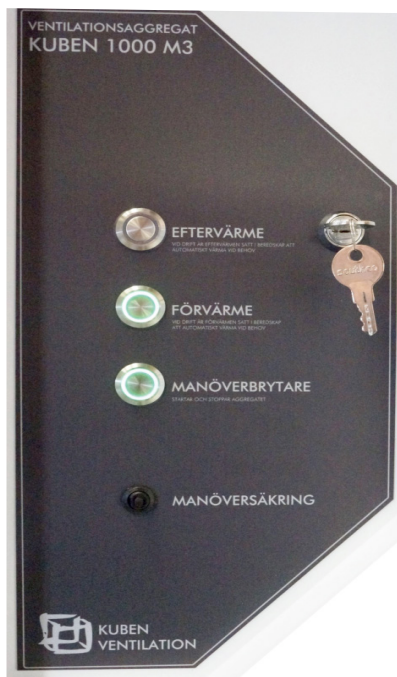
Internal control panel
